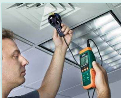
Typical application of measuring air velocity and temperature in HVAC
