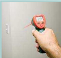
Check building for insufficient insulation
