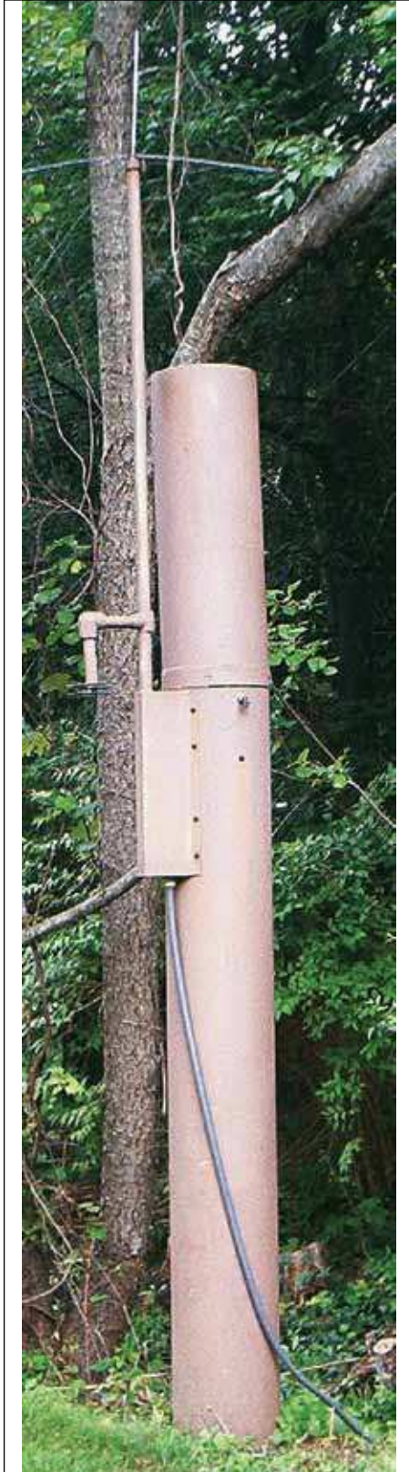
Shown monitoring river level for flood warning.
